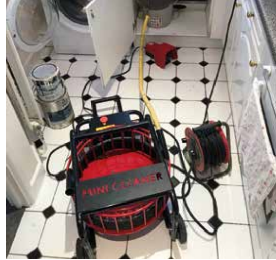
Photo courtesy of MT Drains
